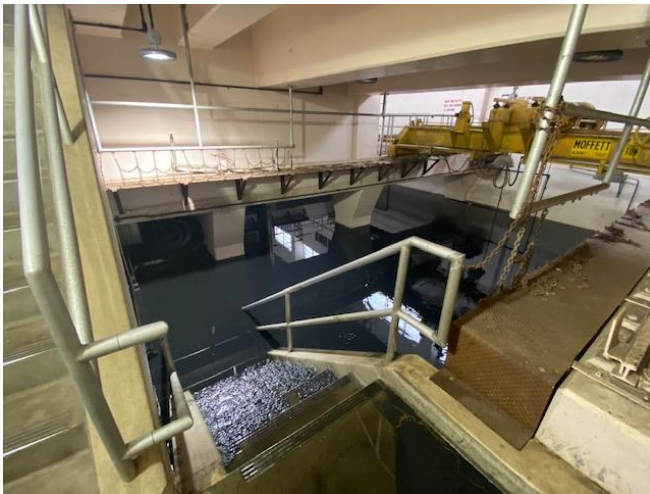
Figure 10: Flood waters in the EPP (Effluent Pumping Plant) basement area.
