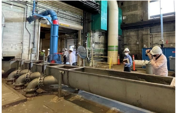
Figure 13: Backside of the sluice showing three pipes from the sluice to the chopper pumps below.
