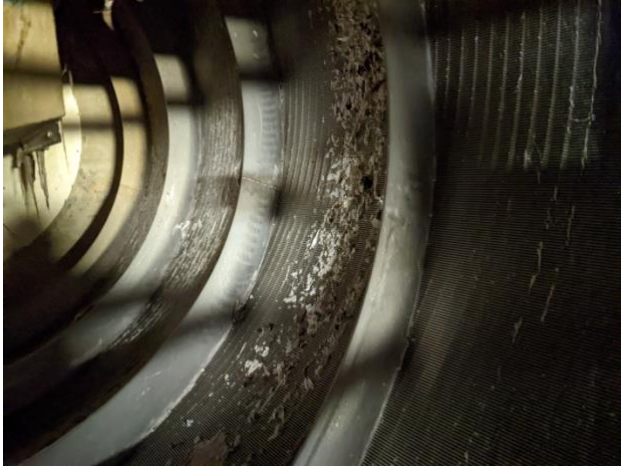
Figure 20: Internal of a drum screen.
