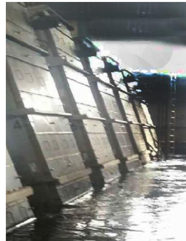
Figure 11: Flood waters in the Headworks building.
